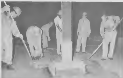
Some spots that need special treatment are the bases of the I-beam supports in the tank. Arston Corporation personnel are doing the job.
